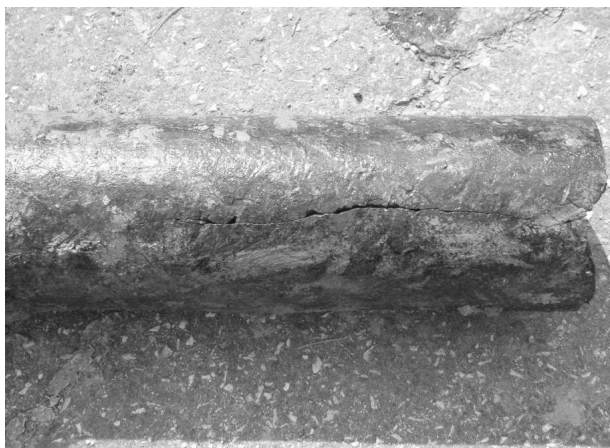
Figure 4. Cracked fragment of water pipeline
